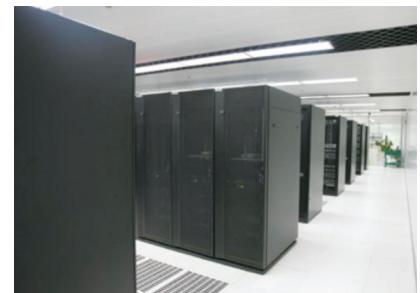
Other IT or Computer Equipment Room
